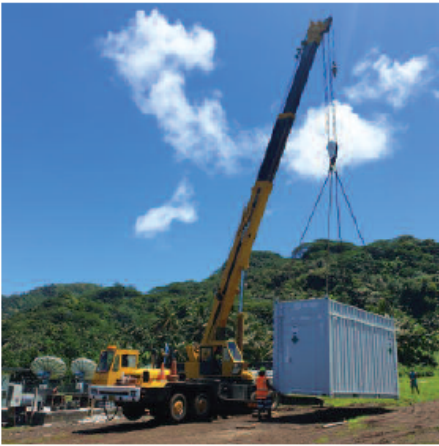
Figure 6: Containerised Cable Landing Station
